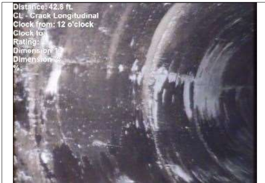
At: 42.8 ft. 12/ CL - Crack Longitudinal Joint: No
