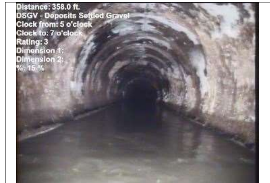
At: 358 ft. 5/7 DSGV - Deposits Settled Gravel Joint: No 15 %
