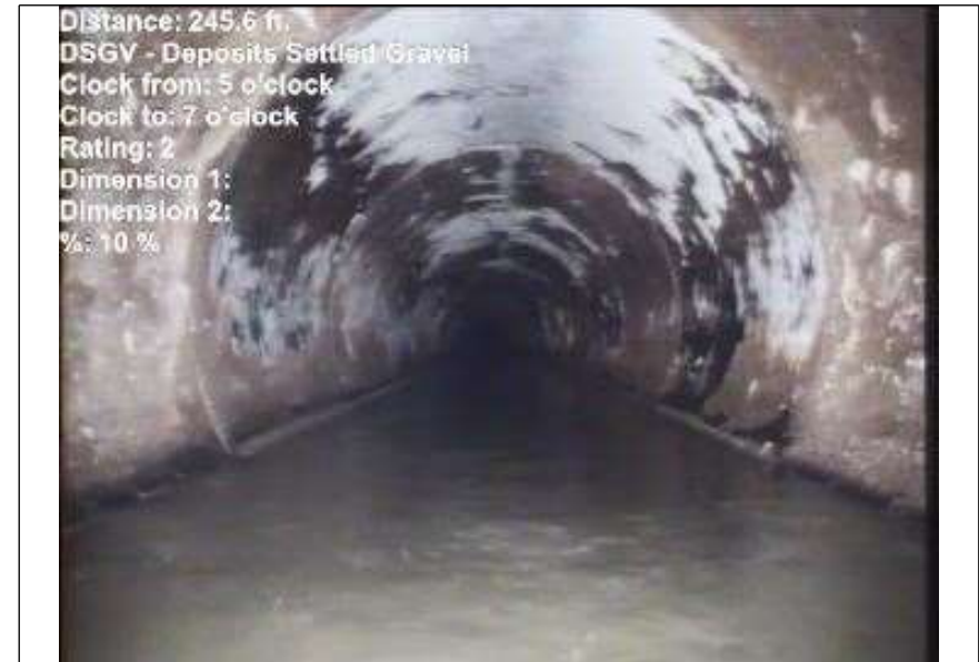
At: 245.6 ft. 5/7 DSGV - Deposits Settled Gravel Joint: No 10 %
