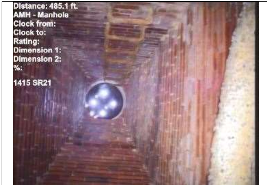
At: 485.1 ft. AMH - Manhole Joint: No 1415 SR21
