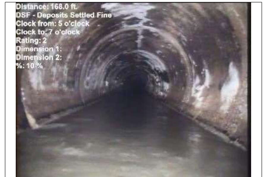
At: 168 ft. 5/7 DSGV - Deposits Settled Gravel Joint: No 10 %
