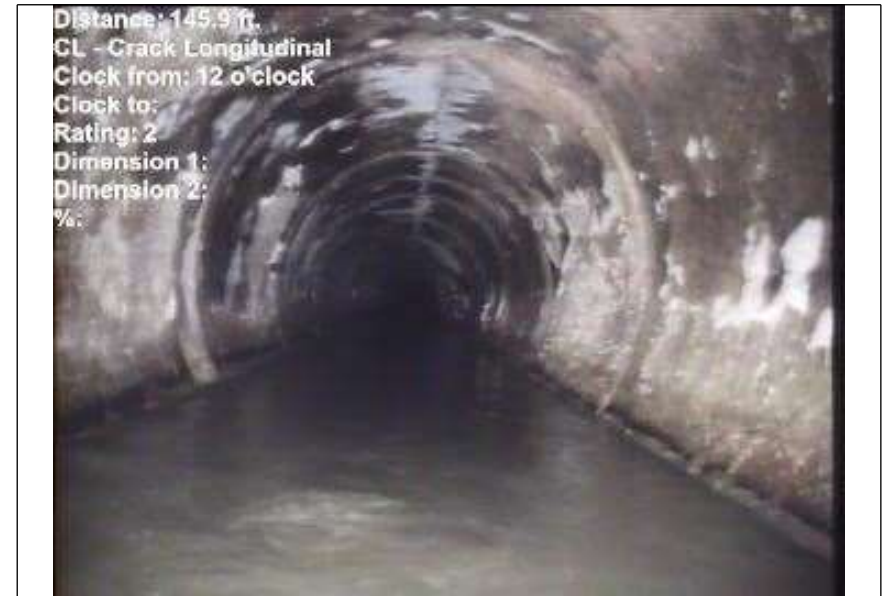
At: 145.9 ft. 12/. CL - Crack Longitudinal Joint: No
