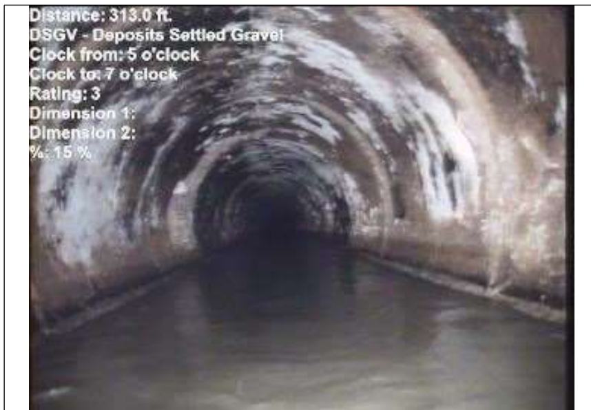
At: 313 ft. 5/7 DSGV - Deposits Settled Gravel Joint: No 15 %
