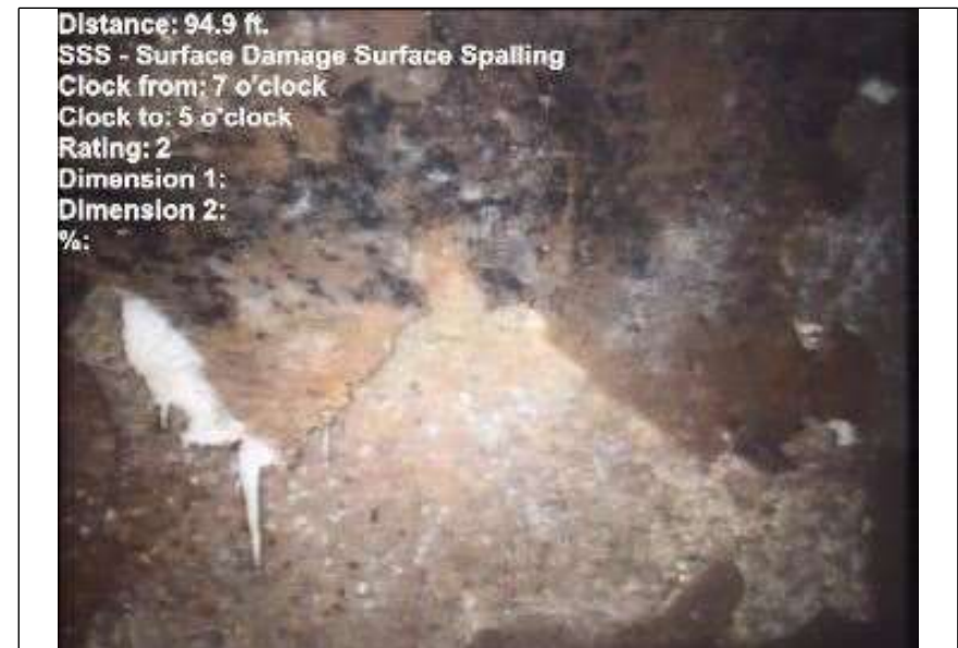
At: 94.9 ft. 7/5 SSS - Surface Damage Surface Spalling Joint: No
