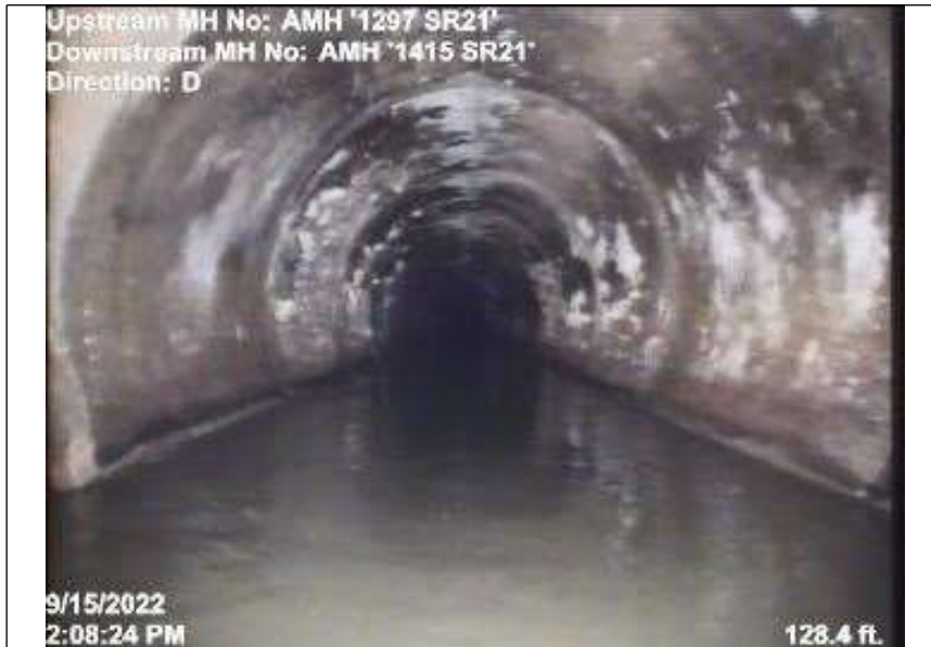
At: 121 ft. 12/. CL - Crack Longitudinal Joint: No
