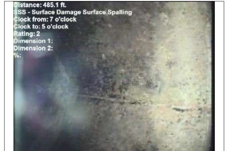
At: 485.1 ft. 7/5 SSS - Surface Damage Surface Spalling Joint: No
