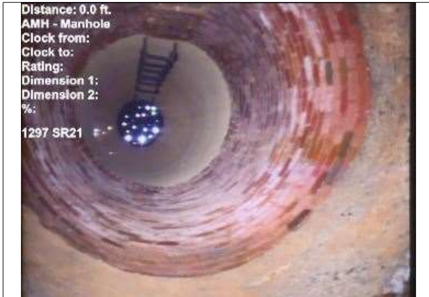
At: 0 ft. AMH - Manhole Joint: No 1297 SR21
