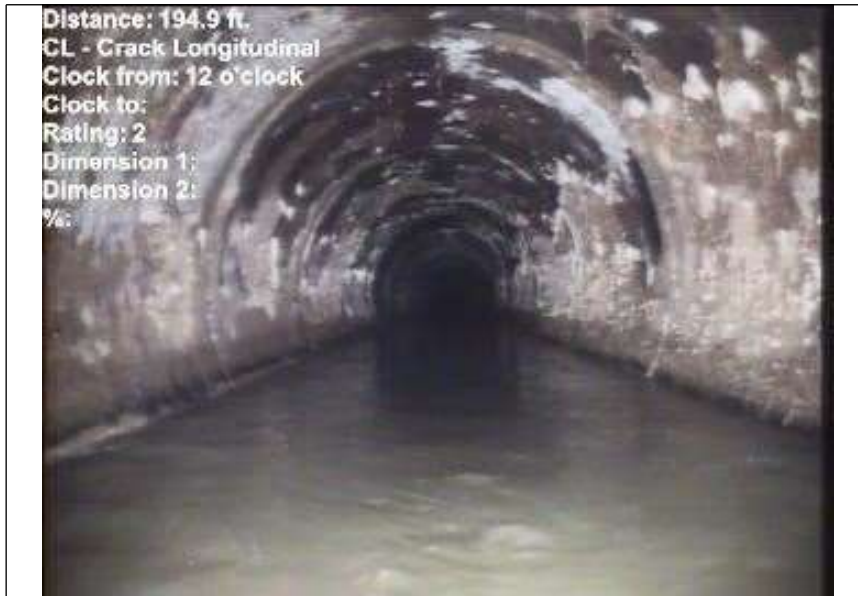
At: 194.9 ft. 12/. CL - Crack Longitudinal Joint: No
