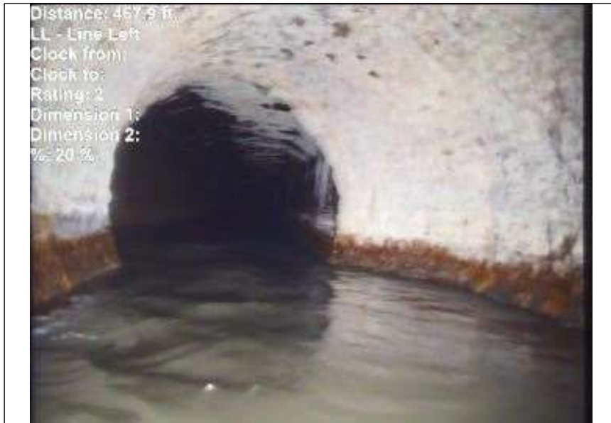
At: 467.9 ft. LL - Line Left Joint: No 20 %
