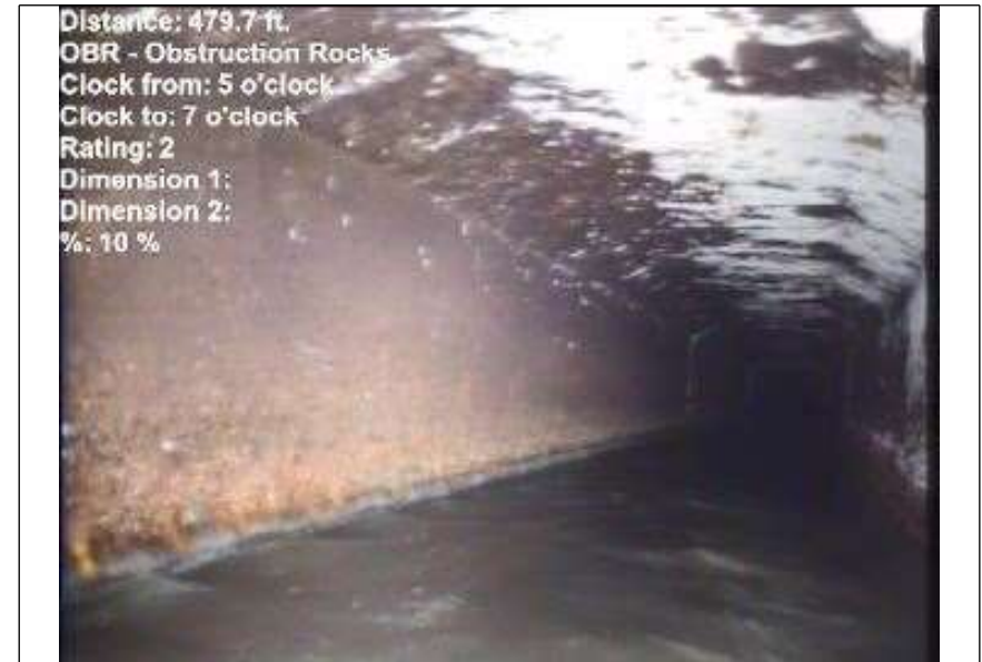
At: 479.7 ft. 5/7 OBR - Obstruction Rocks Joint: No 10 %
