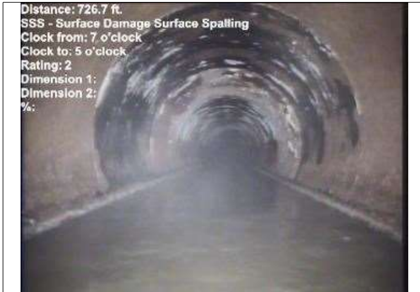
At: 726.7 ft. 7/5 SSS - Surface Damage Surface Spalling Joint: No
