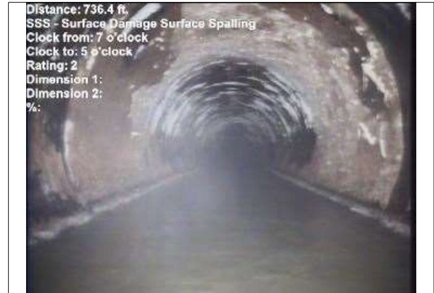
At: 736.4 ft. 7/5 SSS - Surface Damage Surface Spalling Joint: No
