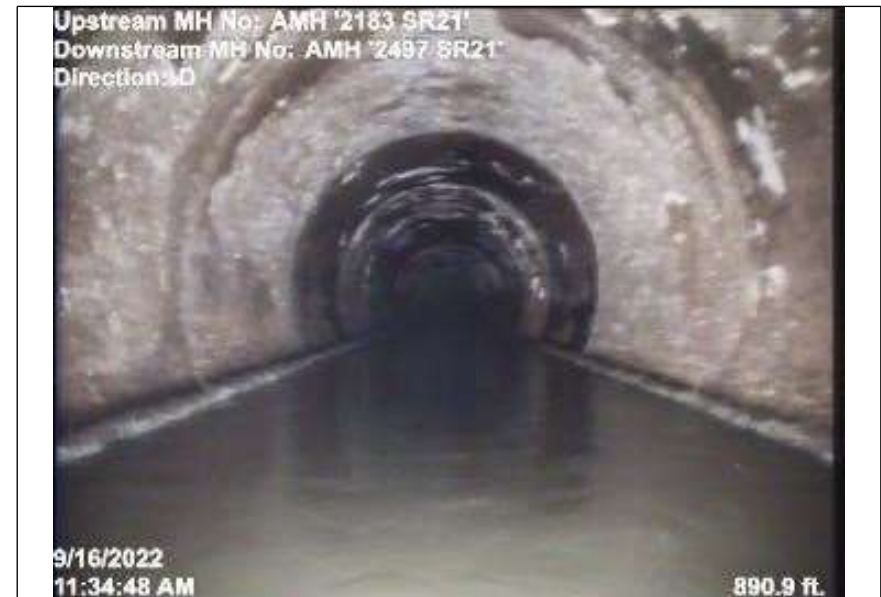
At: 883.5 ft. 7/5 SSC - Surface Spalling of Damage Coating Joint: No
