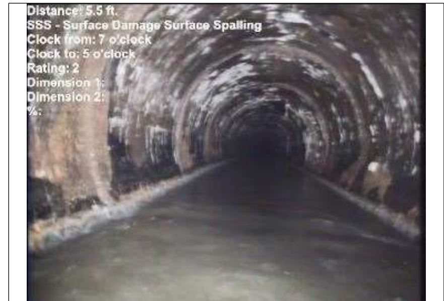
At: 5.5 ft. 7/5 SSS - Surface Damage Surface Spalling Joint: No
