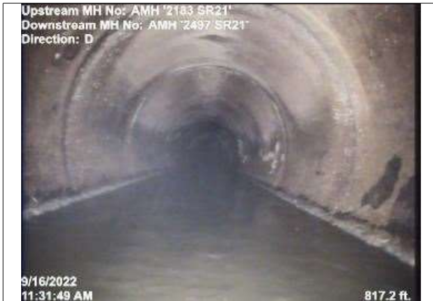
At: 816.2 ft. 7/5 SSS - Surface Damage Surface Spalling Joint: No
