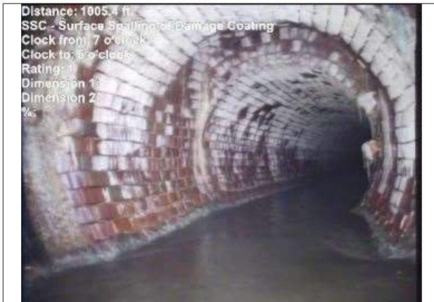
At: 1005.4 ft. SSC - Surface Spalling of Damage Coating 7/5
