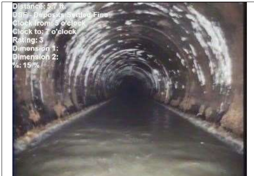
At: 5.7 ft. 5/7 DSF - Deposits Settled Fine Joint: No 15 %
