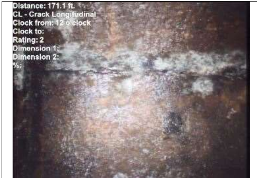
At: 171.1 ft. 12/. CL - Crack Longitudinal Joint: No
