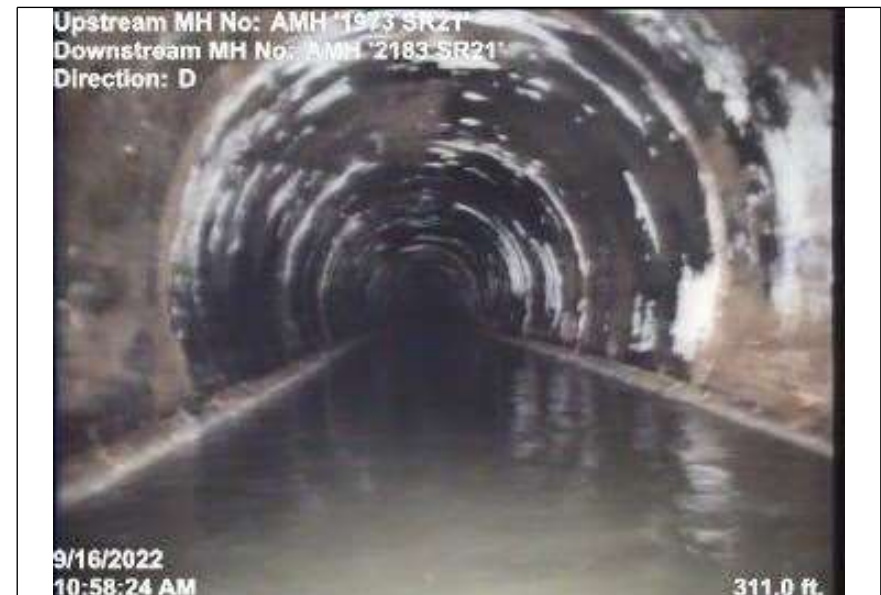
At: 305.4 ft. 12/. CL - Crack Longitudinal Joint: No
