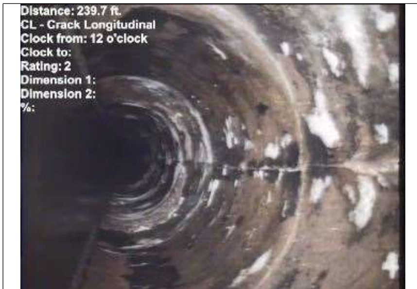
At: 239.7 ft. 12/. CL - Crack Longitudinal Joint: No
