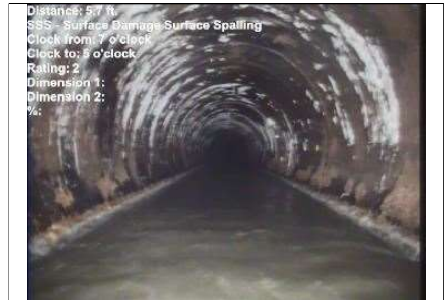
At: 5.7 ft. 7/5 SSS - Surface Damage Surface Spalling Joint: No
