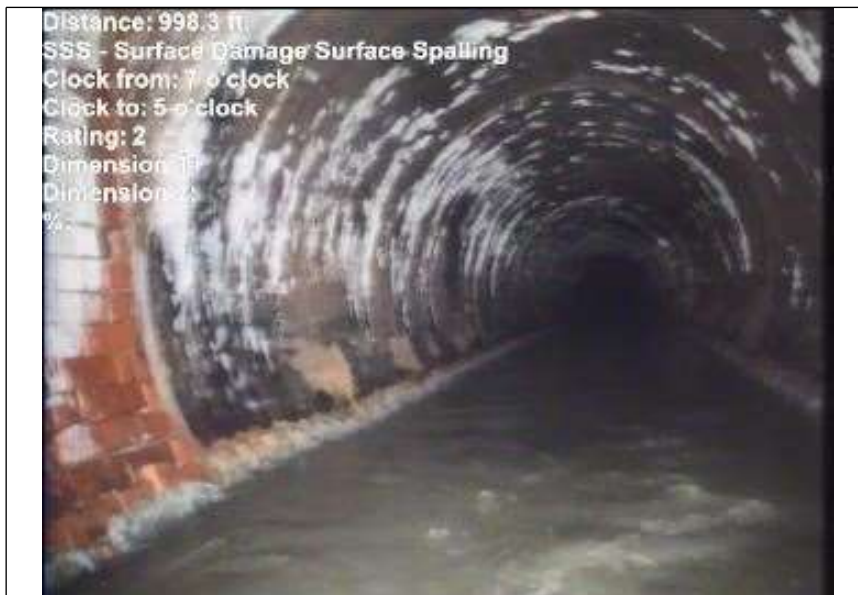
At: 998.3 ft. 7/5 SSS - Surface Damage Surface Spalling Joint: No
