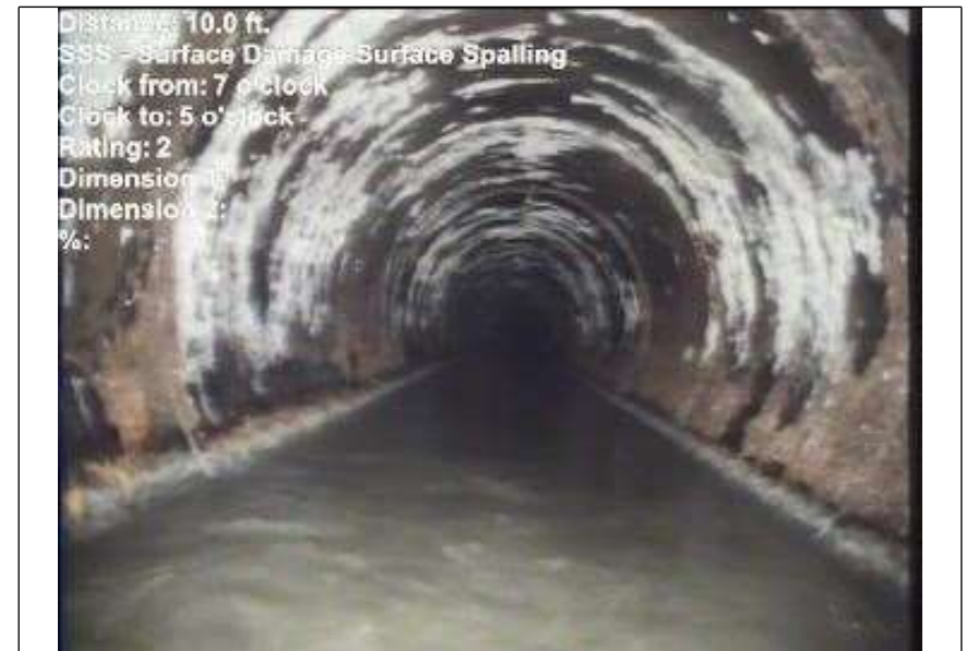
At: 10 ft. 7/5 SSS - Surface Damage Surface Spalling Joint: No
