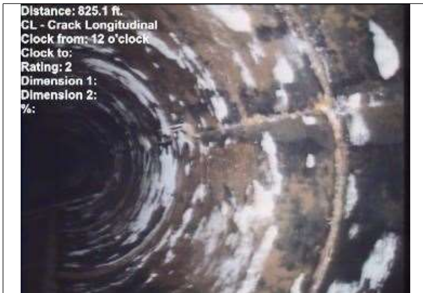
At: 825.1 ft. 12/. CL - Crack Longitudinal Joint: No
