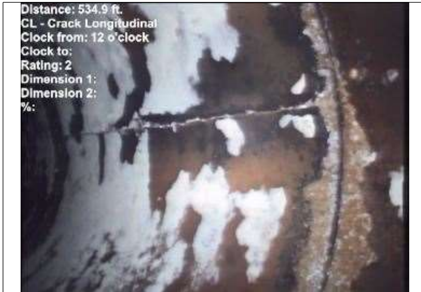
At: 534.9 ft. 12/ CL - Crack Longitudinal Joint: Yes
