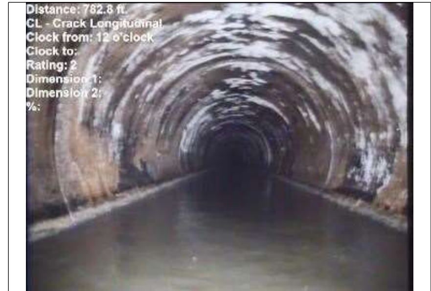
At: 782.8 ft. 12/. CL - Crack Longitudinal Joint: No
