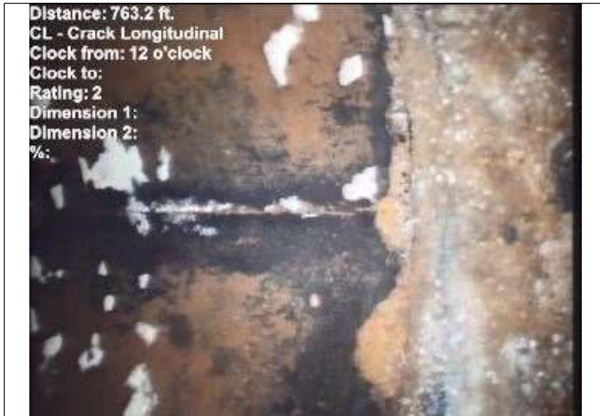
At: 763.2 ft. 12/. CL - Crack Longitudinal Joint: No
