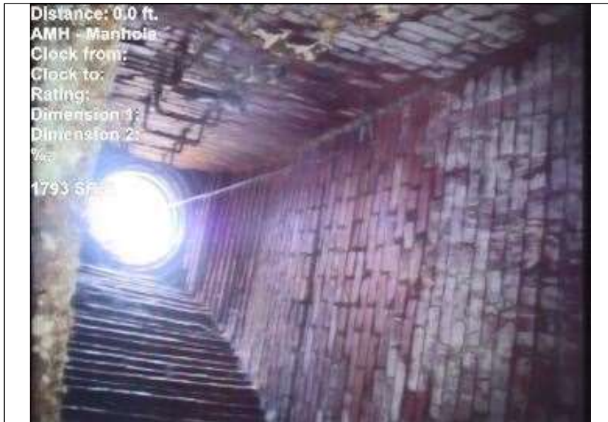
At: 0 ft. AMH - Manhole Joint: No 1793 SR21
