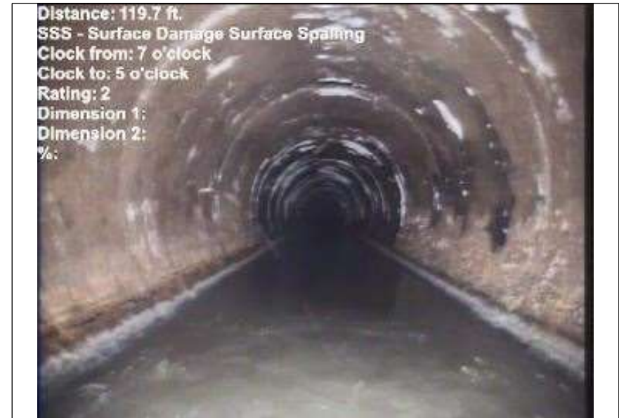
At: 119.7 ft. 7/5 SSS - Surface Damage Surface Spalling Joint: No
