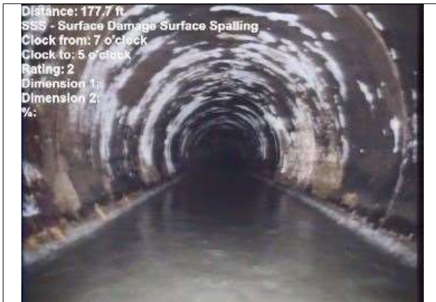
At: 177.7 ft. 7/5 SSS - Surface Damage Surface Spalling Joint: No
