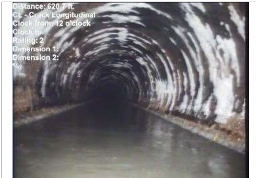
At: 620.7 ft. 12/ CL - Crack Longitudinal Joint: Yes
