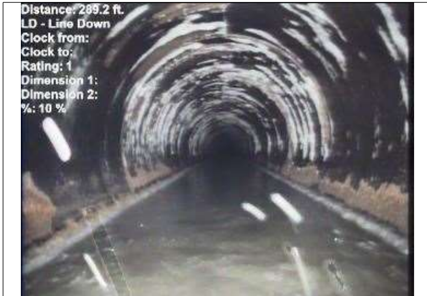
At: 289.2 ft. LD - Line Down Joint: No 10 %
