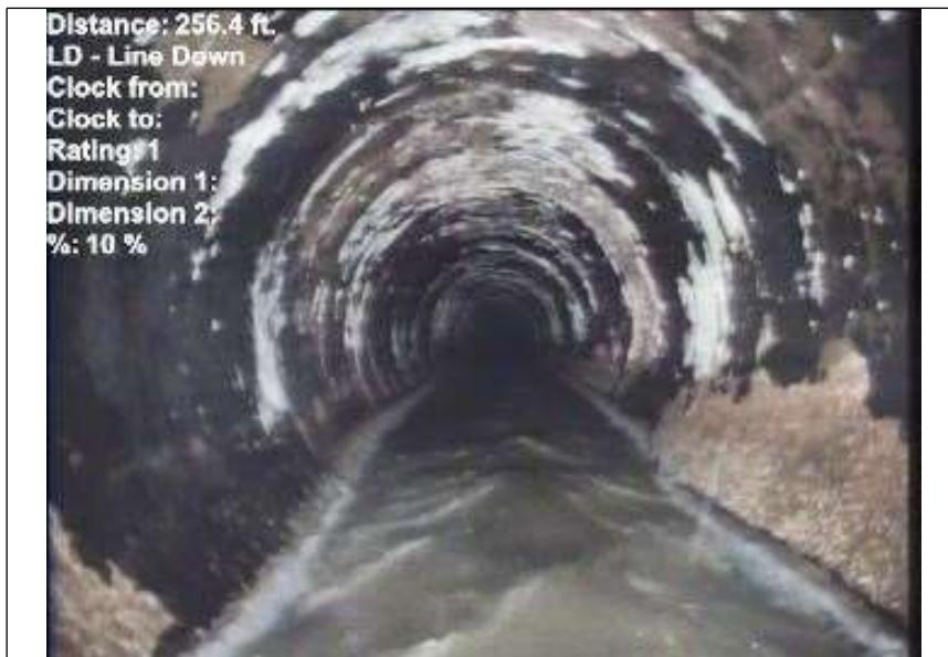
At: 256.4 ft. LD - Line Down Joint: No 10 %
