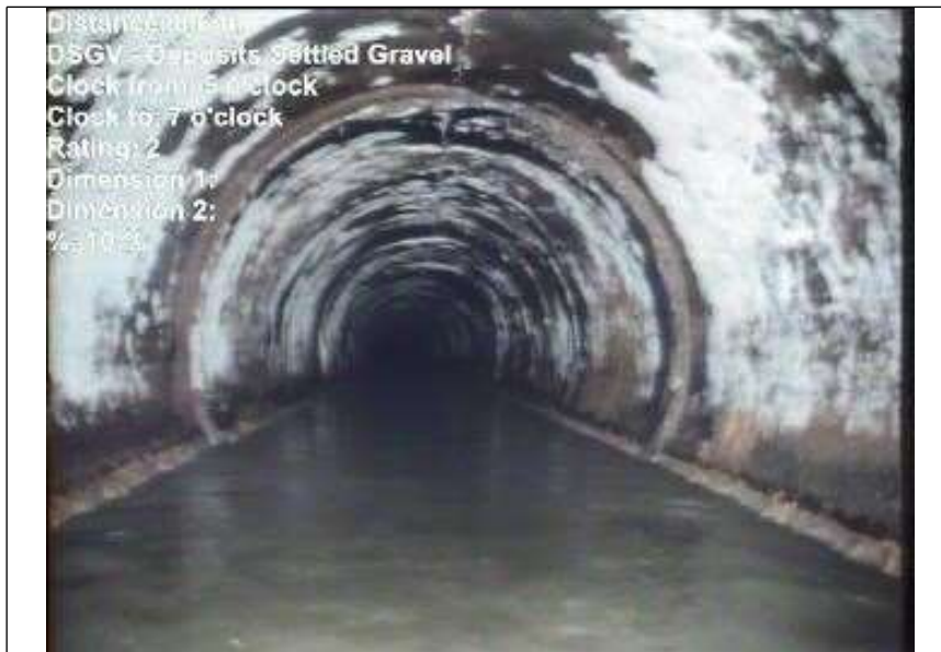
At: 8.6 ft. 5/7 DSGV - Deposits Settled Gravel Joint: No 10 %
