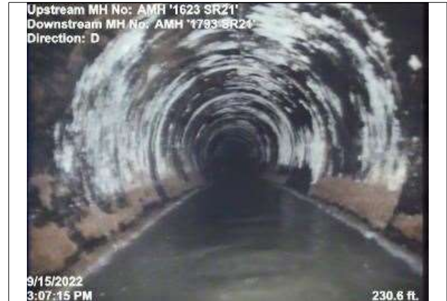
At: 227 ft. 12/. CL - Crack Longitudinal Joint: No
