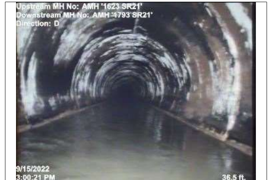
At: 32.9 ft. 5/7 DSGV - Deposits Settled Gravel Joint: No 10 %
