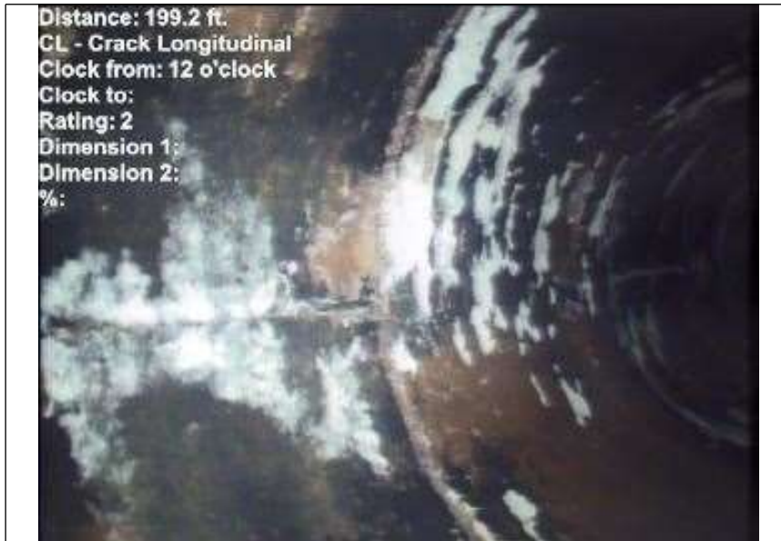
At: 199.2 ft. 12/. CL - Crack Longitudinal Joint: No
