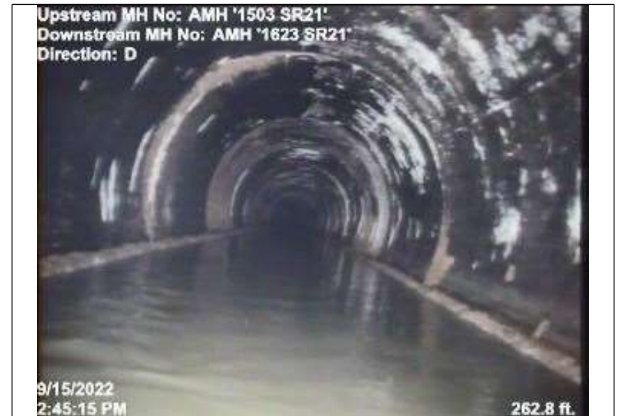
At: 260.6 ft. 5/7 DSGV - Deposits Settled Gravel Joint: No 15 %
