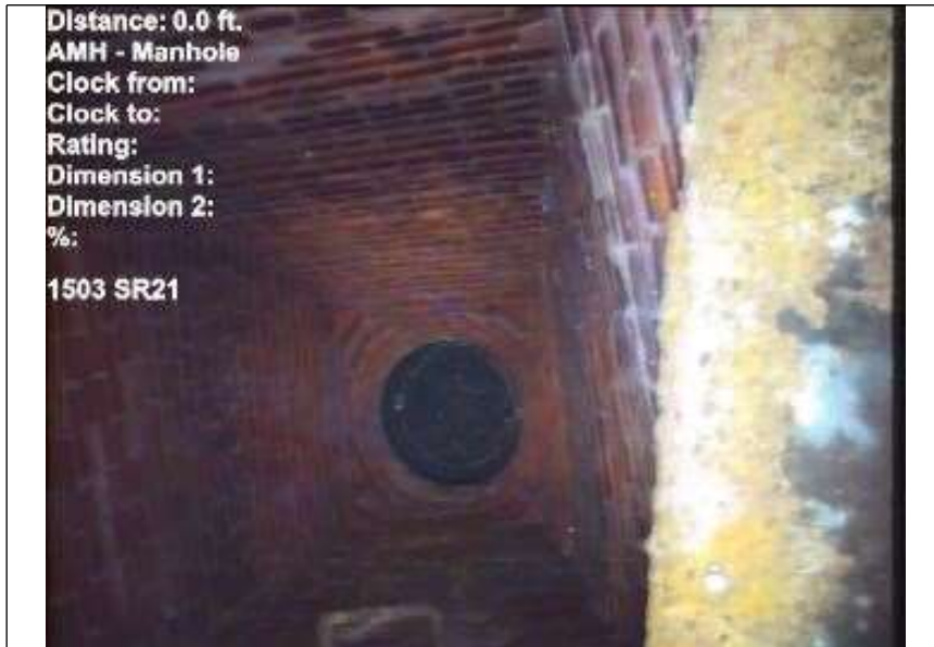
At: 0 ft. AMH - Manhole Joint: No 1503 SR21
