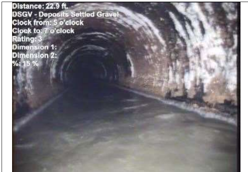
At: 22.9 ft. 5/7 DSGV - Deposits Settled Gravel Joint: No 15 %
