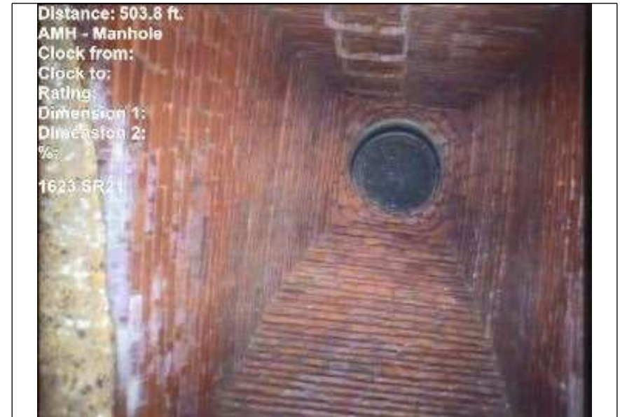
At: 503.8 ft. AMH - Manhole Joint: No 1623 SR21
