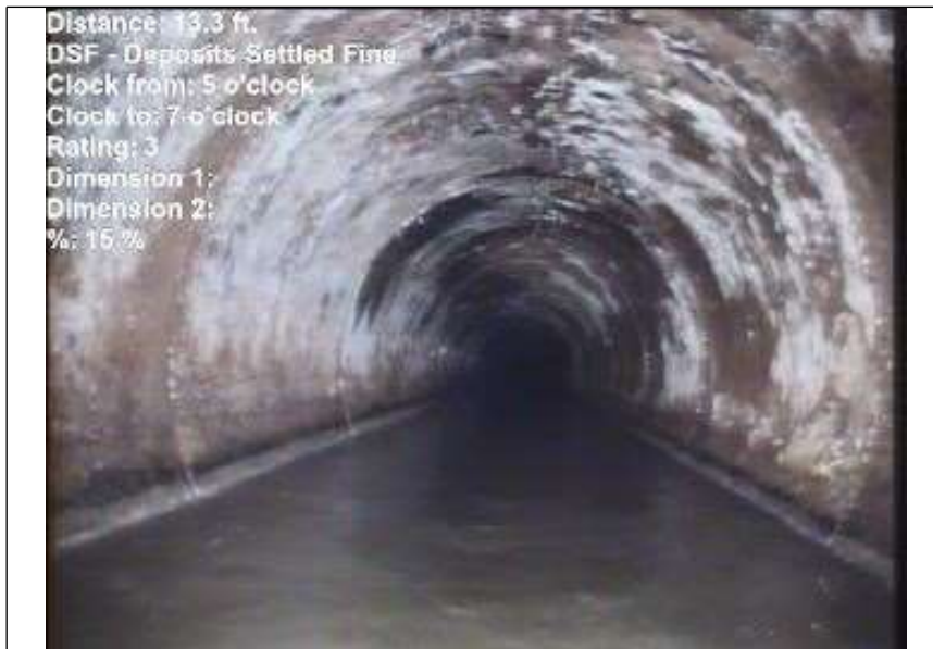
At: 13.3 ft. 5/7 DSF - Deposits Settled Fine Joint: No 15 %
