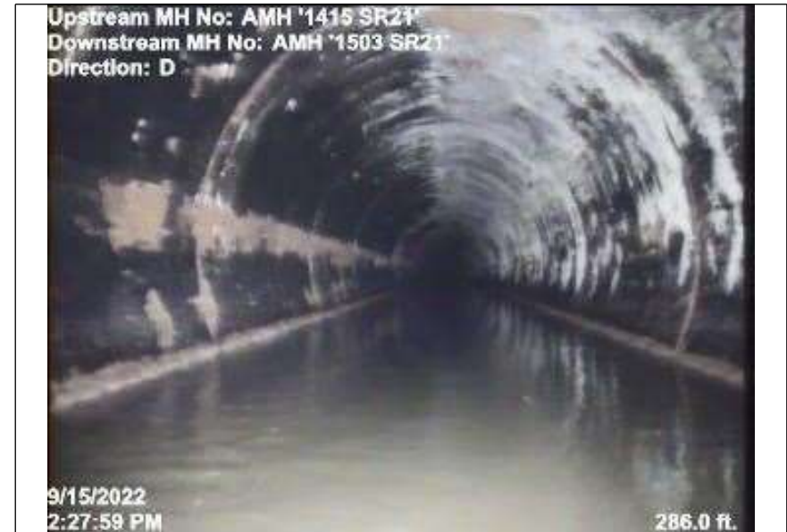
At: 282.4 ft. 5/7 DSF - Deposits Settled Fine Joint: No 15 %
