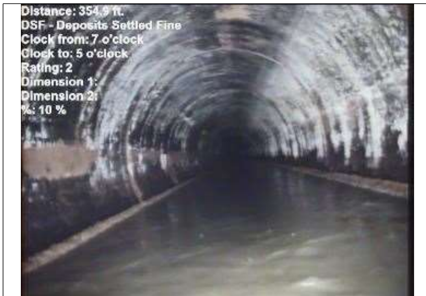
At: 354.9 ft. 7/5 DSF - Deposits Settled Fine Joint: No 10 %
