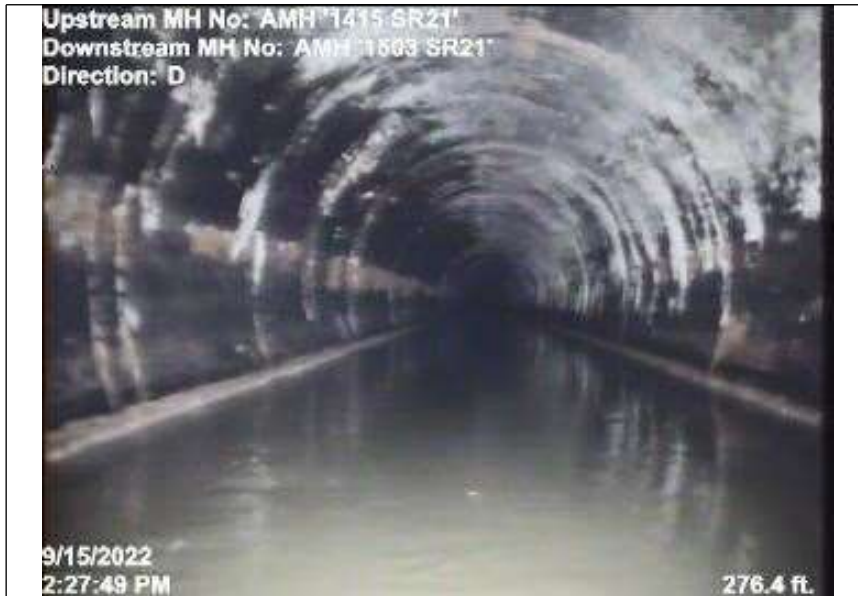
At: 273 ft. 7/5 SSC - Surface Spalling of Damage Coating Joint: No
