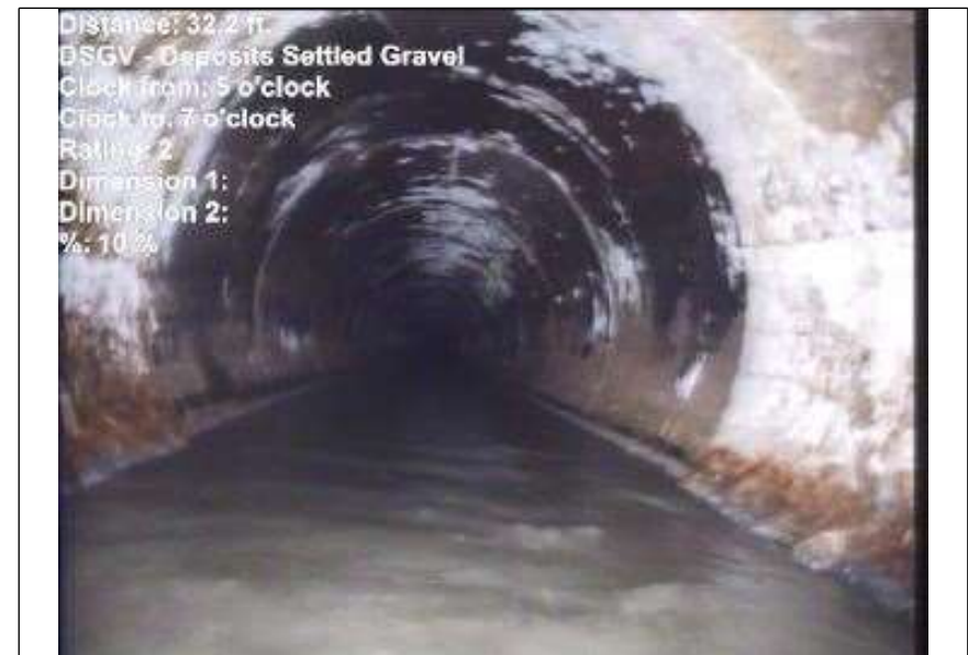
At: 32.2 ft. 5/7 DSGV - Deposits Settled Gravel Joint: No 10 %
