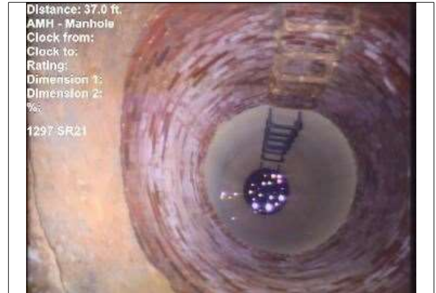
At: 37 ft. AMH - Manhole Joint: No 1297 SR21
