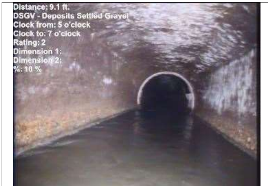
At: 9.1 ft. 5/7 DSGV - Deposits Settled Gravel Joint: No 10 %
