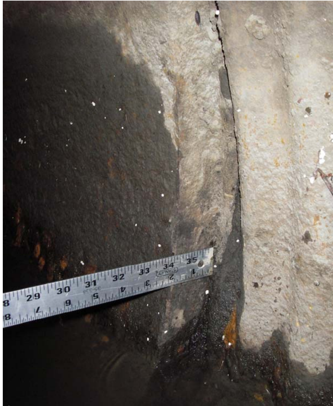
Offset joint at 4:00 where CMP meets RCP (approx. 2")
