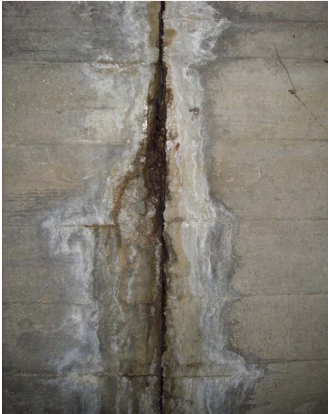
Weeping joint, exposed rebar at right side-56ft
