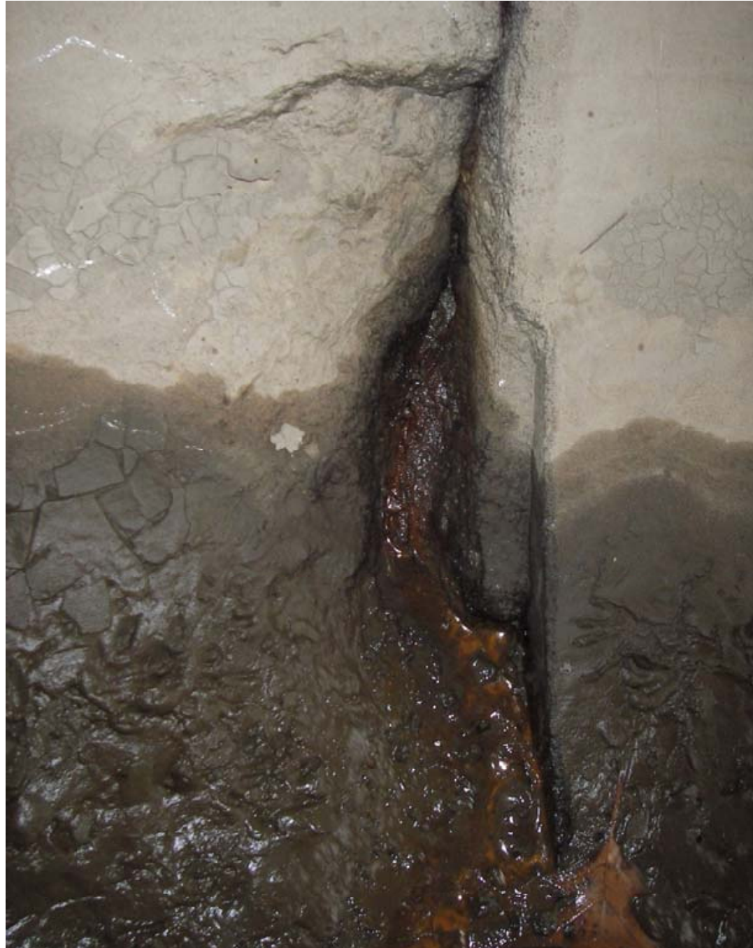
Scouring at joint in left haunch/soil or rust seeping in through joint- 79ft
