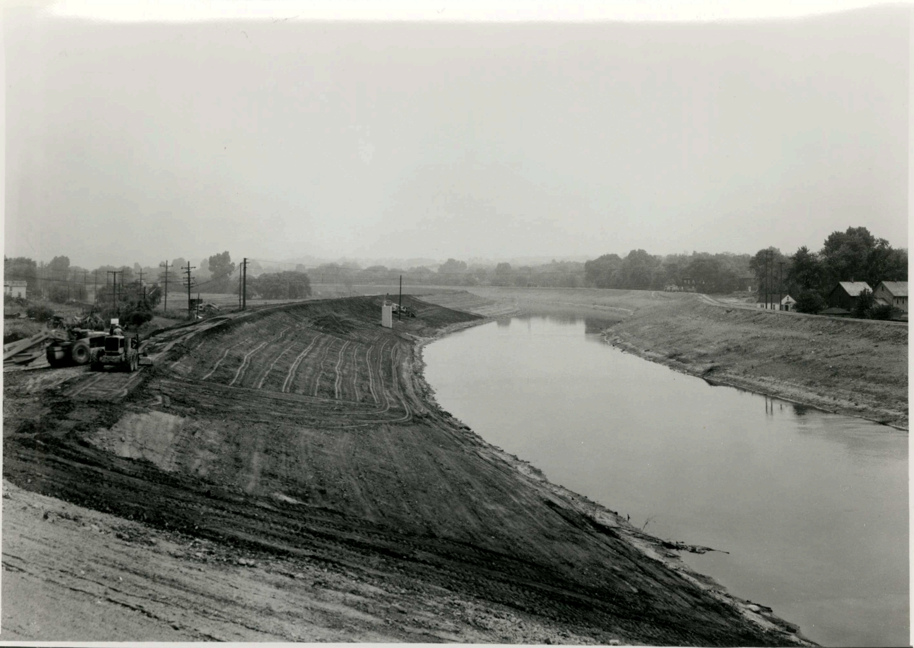
Cherry Road at Station 8+50 looking upstream showing construction of new channel and levee embankment
