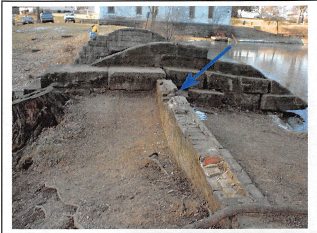
View of the brick cut-off wall across the left half of crest. The blue arrow indicates where bricks have become displaced from the wall.
