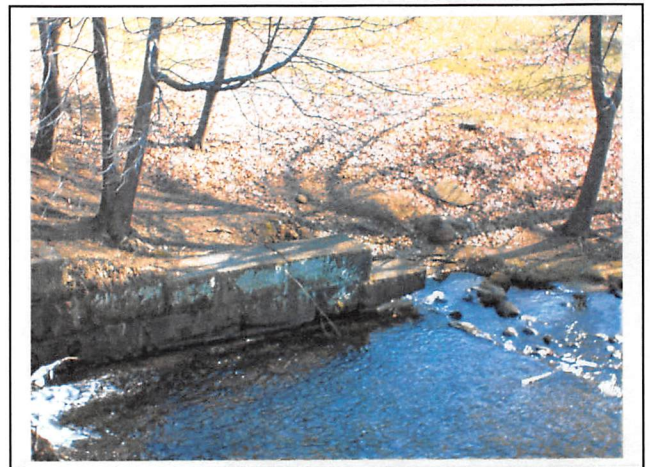
Other views of the undermining and erosion at the downstream end of the left side wall.
