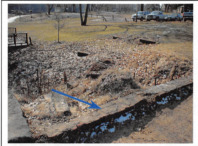
View of the brick cut-off wall across the right half of crest and the downstream slope.
