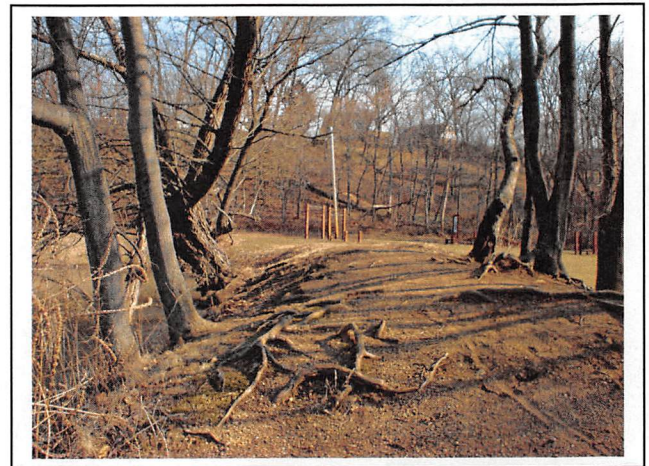
View of the left crest. Note the lack of vegetal cover and the exposed tree roots from erosion.
