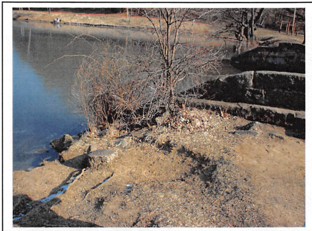
View of the right upstream slope and crest near the principal spillway inlet. Note the erosion and lack of vegetal ground cover.
