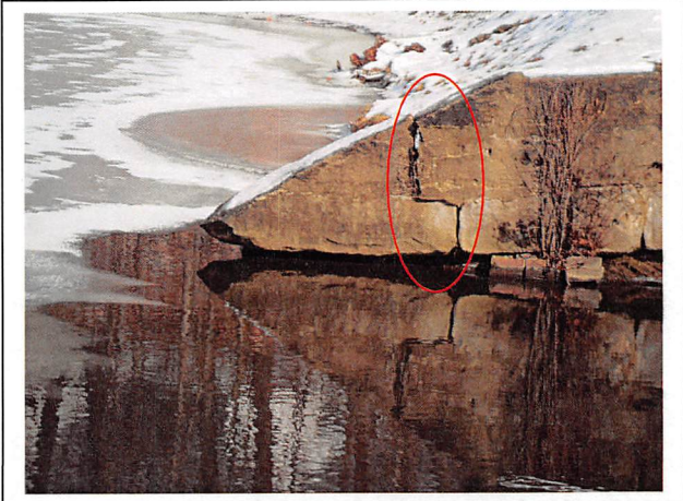
View of the upstream end of the left principal spillway wall in 2016. Note that the stones have shifted and now daylight can be seen between the stones.
