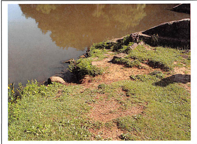
View of the upstream slope that abuts the right principal spillway sidewall in 2010.
