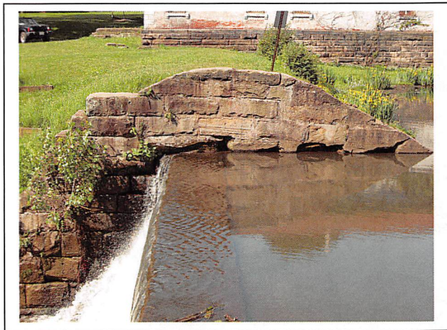
View of the right principal spillway side wall in June 2010. This wall has remained for the most part unchanged.
