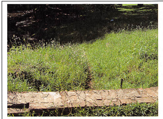
View of the brick cutoff wall on the right side of the spillway in 2010. Note that the wall is intact. (View from upstream to downstream)
