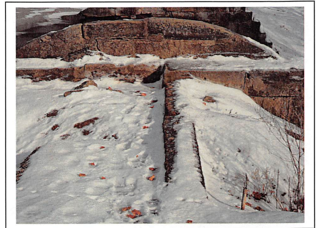
View of the brick cutoff wall on the right side of the spillway in 2016. Note that the wall has remained intact. (View from right to left)
