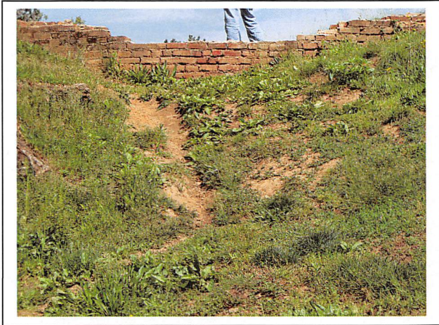
View of the brick cutoff wall on the left side of the spillway in 2010. Note that the bricks are becoming displaced.
