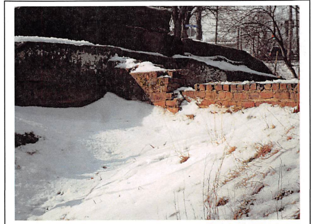
View of the brick cutoff wall on the left side of the spillway in 2016. Note that another layer of bricks has been displaced.
