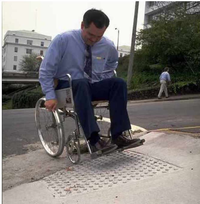
Figure 8-18. Photo. A pavement grinding project left an exaggerated lip at this curb cut.
