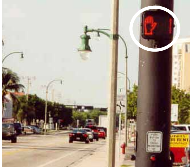
Figure 10-12. Photo. Example of countdown pedestrian signal in Lauderdale-By-The-Sea, FL.
