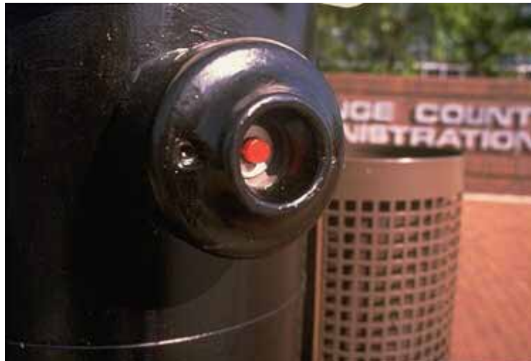
Figure 11-12. Photo. Example of obscure pedestrian pushbuttons; pushbuttons should be conveniently placed and clear from obstacles.
